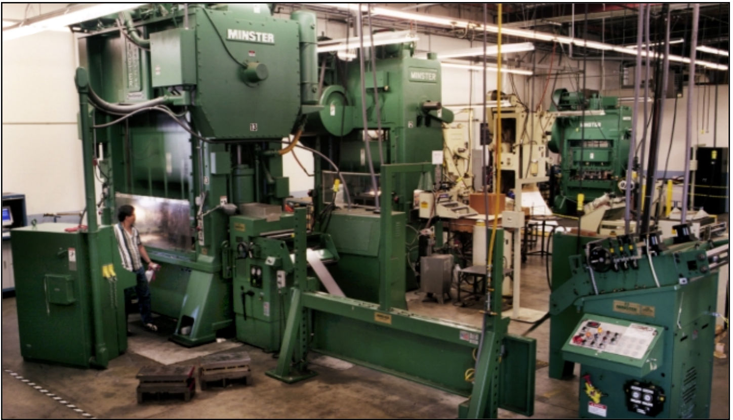
This E2 200 and Minster material handling system is one of the newest additions on Galgon Industry's stamping floor.
